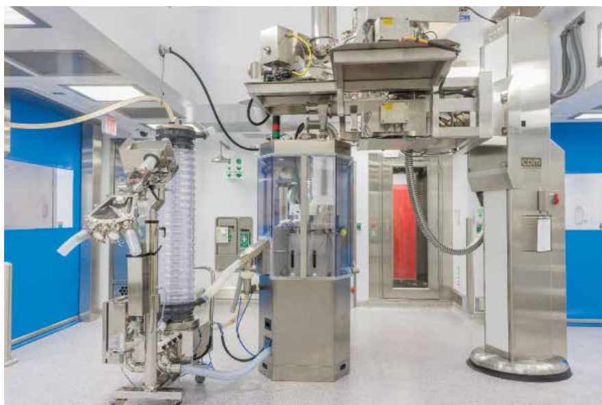
Photo 1: The continuous direct compression suite including gravimetric feeders is mounted on a custom lift assembly to ease access, cleaning, and product changeover.
