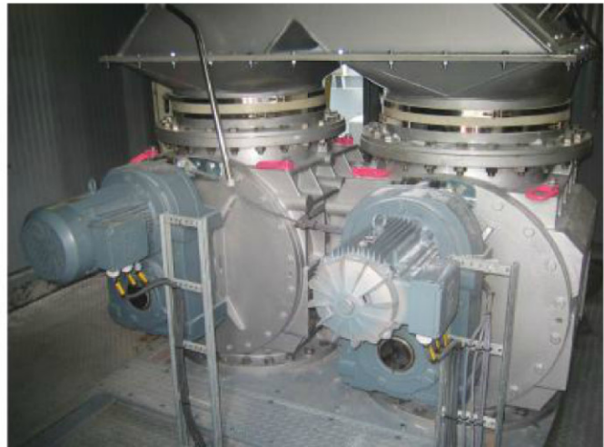
Figure 10: Vacuum ship unloader and rotary valve station.
