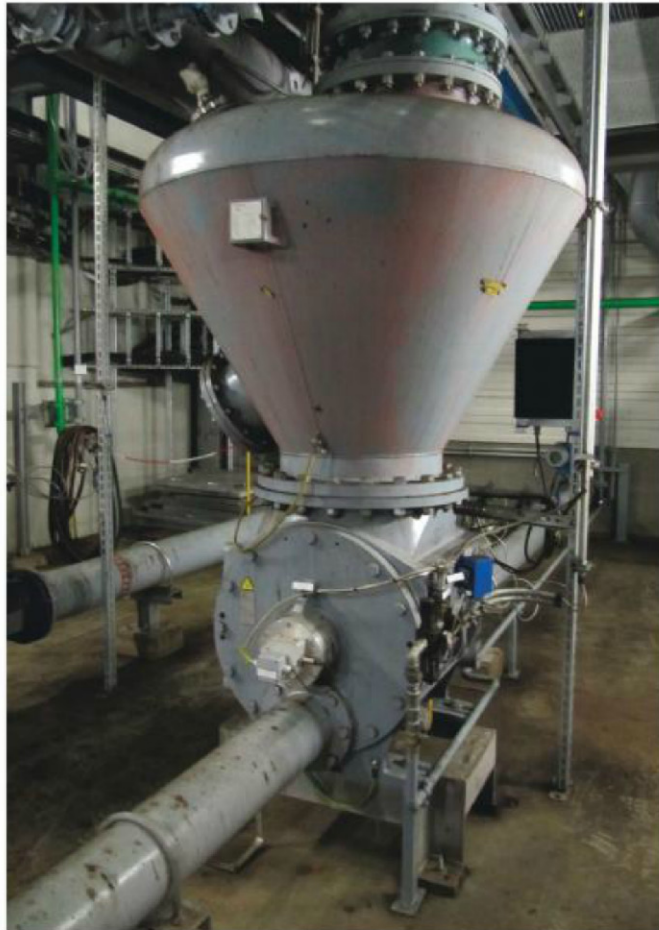
Figure 11: ZXQ 600 for lignite conveying.
